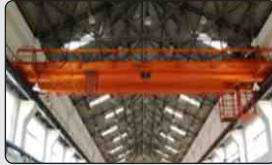
Overhead EOT Crane
